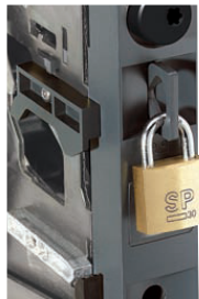
“Disconnected” position locking by padlock.
